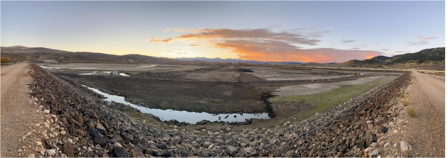
Work began on the Colorado River Connectivity Channel in 2022 at Windy Gap Reservoir.
